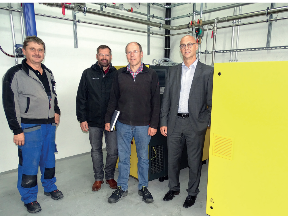
03 The efficiency project was completed this year with the investment in new compressors completed
