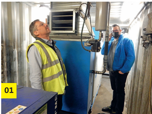
01 One of four compressed-air stations across the site.
